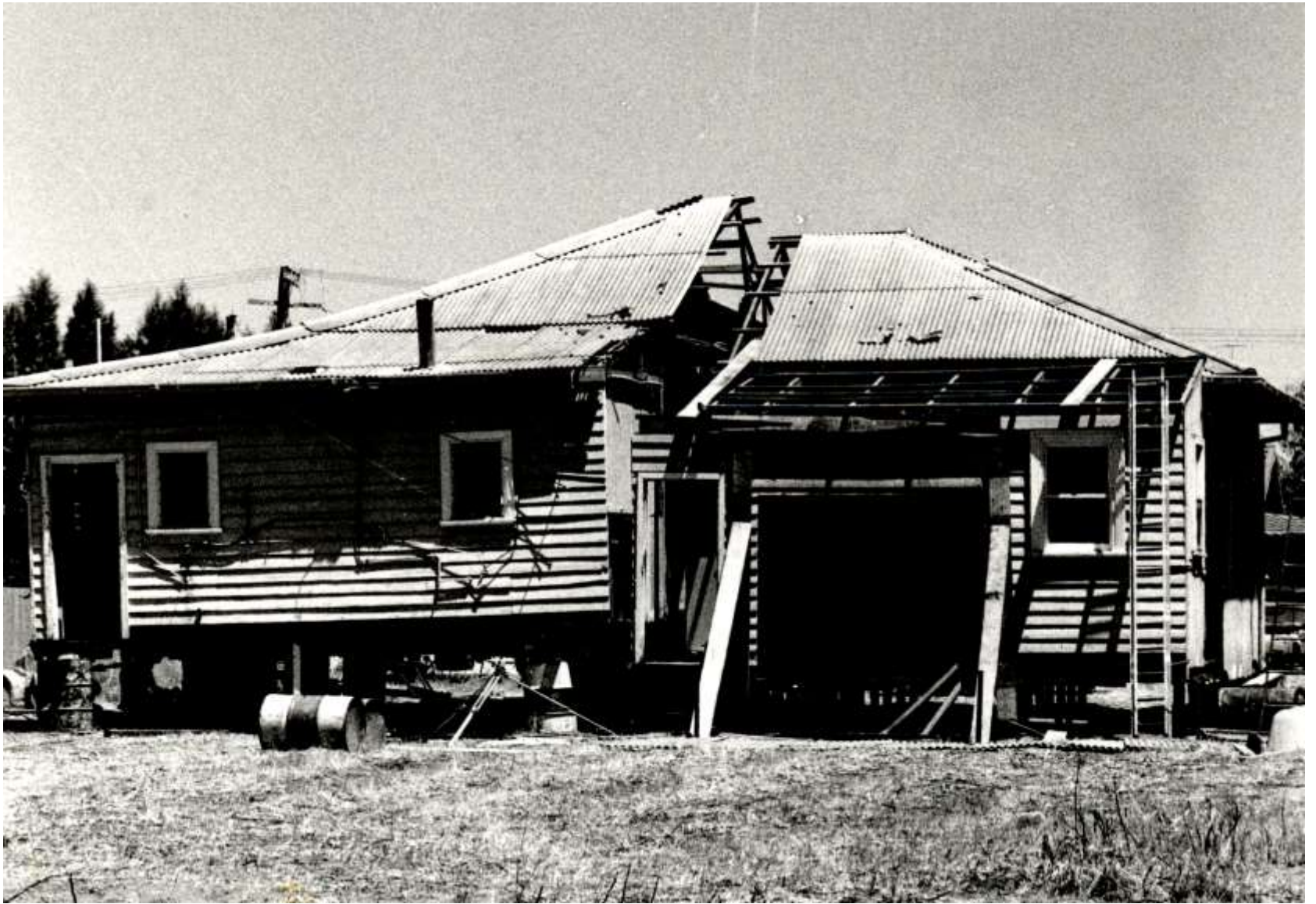
4922: HOME IN BLUFF POINT WITH SEVERE DAMAGE CAUSED TO IT 1983
